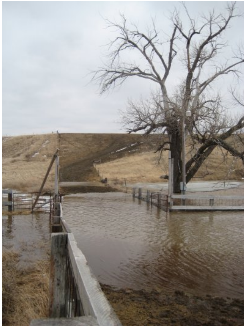
The following picture is the spillway on the dam south of the house. The culvert took all the water it could take, eventually, the water had to escape
